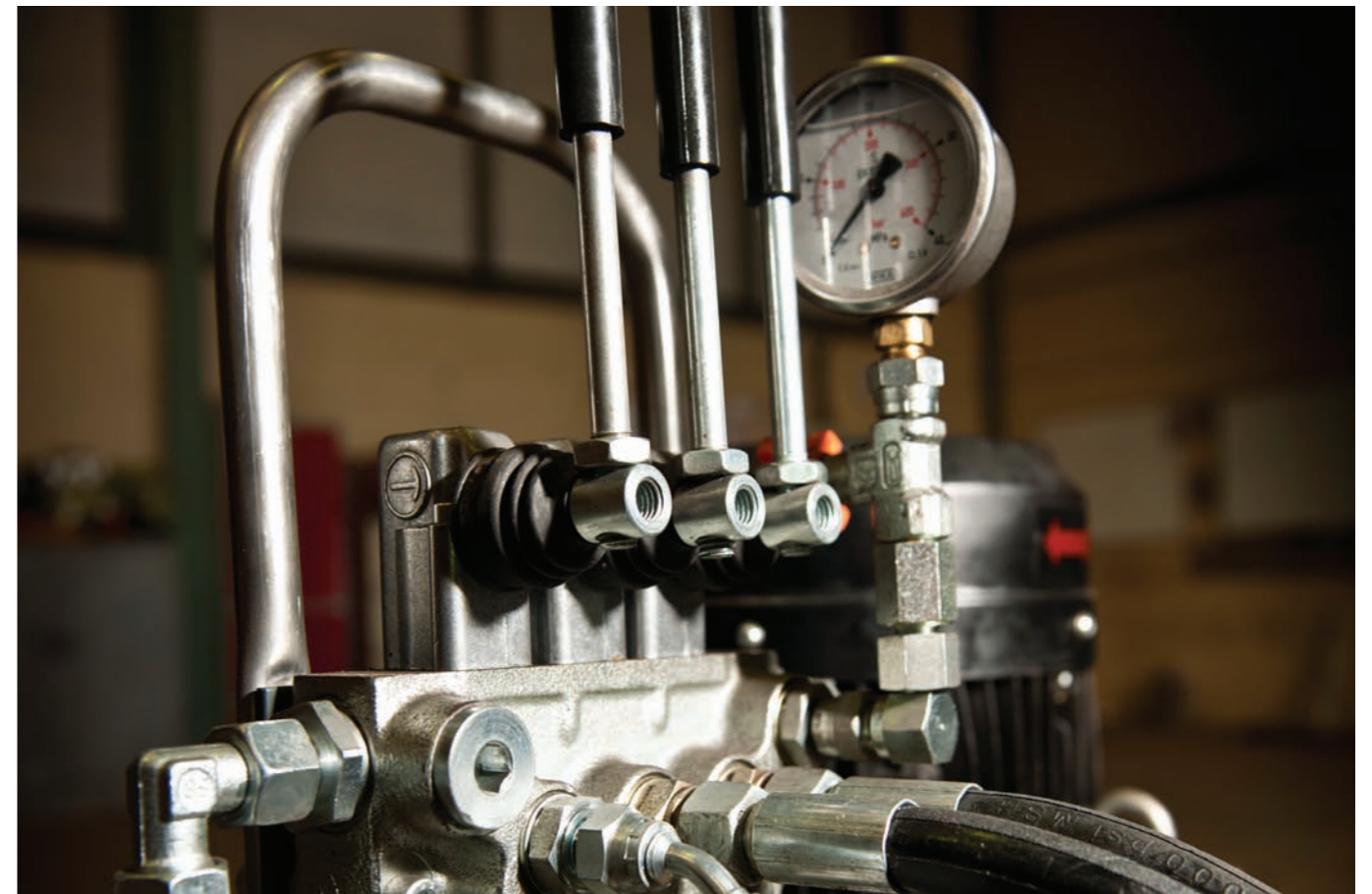
Hydraulic Curtain Adjustment and Frame Opening
